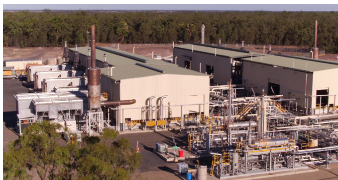
Daandine Power Station
